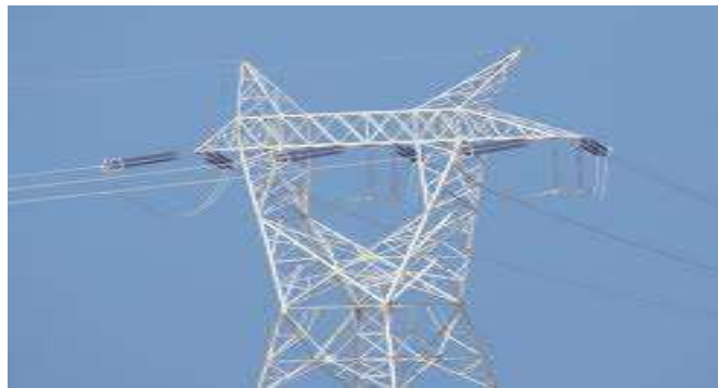
Figure (2) Tension transmission tower
