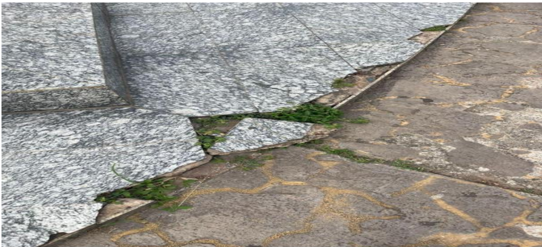
Figure 2: Broken tiles in JJC park.
