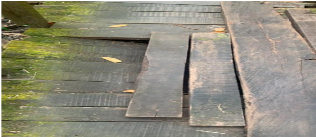
Figure 1: Damaged walkway in Lekki Conservation Center
