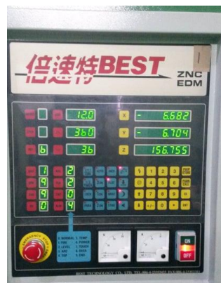
Fig. 9 Feed data in control
